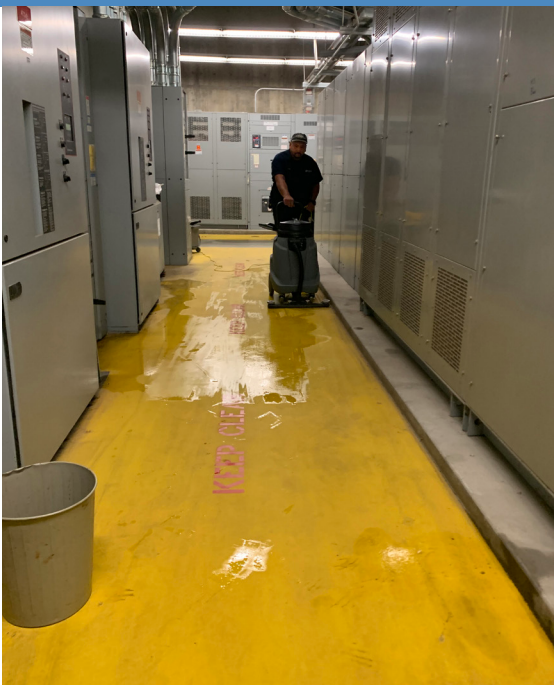
Lead Sr. Custodian Glenn Franco mops standing water in the electrical corridor. (UCR/Angela De La Cruz)
