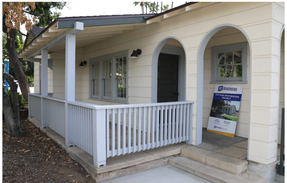
The restored exterior of the University Cottage features fresh paint, a new roof, and an inviting porch that highlights its historical charm. (UCR/Erin Chapman)
