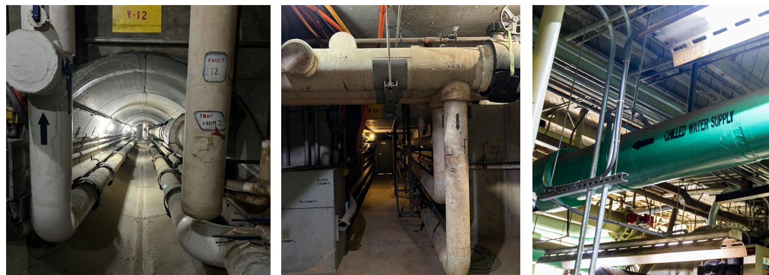
Figure 2-11: Chilled Water Piping in Tunnels
