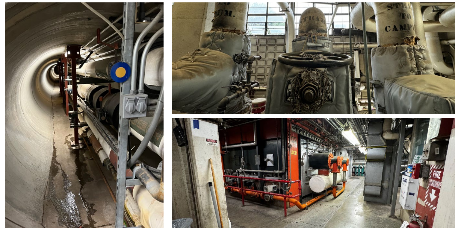
Figure 2-8: Photographs of the Central Utility Plant
