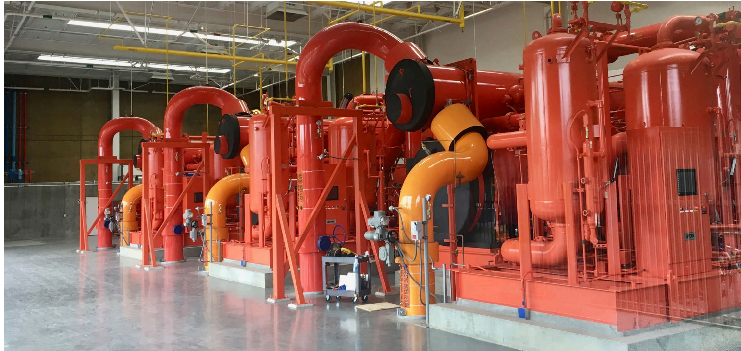
Figure 3-2: Example of WWHP Units 13
